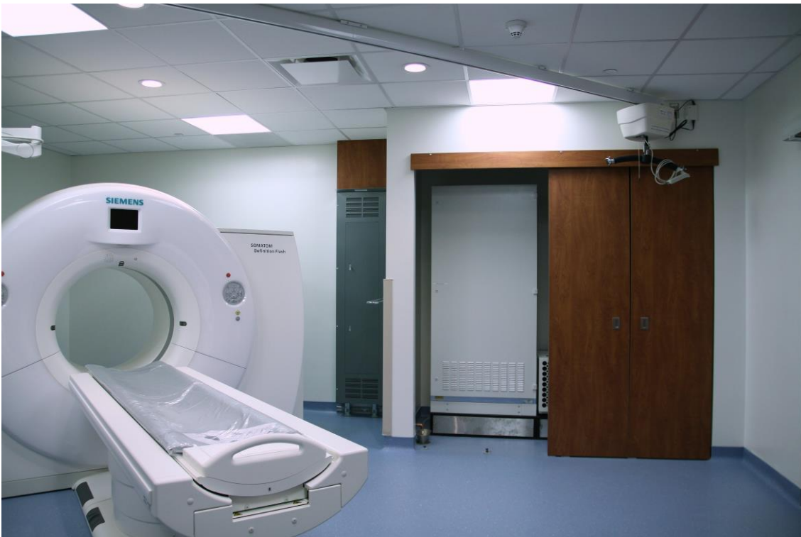
Room view from control window wall.
