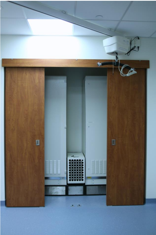
Equipment closet and sliding doors.
