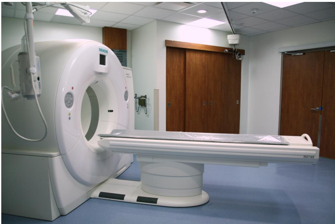
CT, ceiling injector and patient lift all installed.
